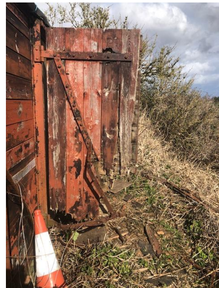
Rear doors damaged.
